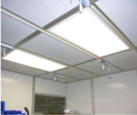
Room System Ionization (Ceiling Grid)
