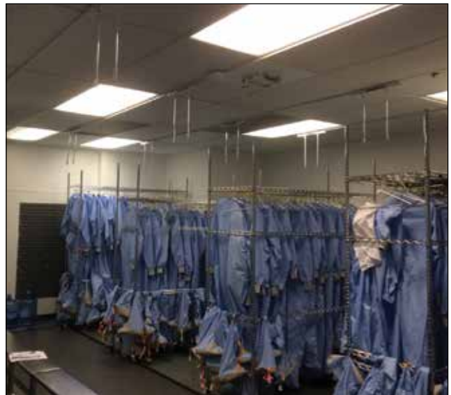
Ceiling Emitters in Gowning Room
