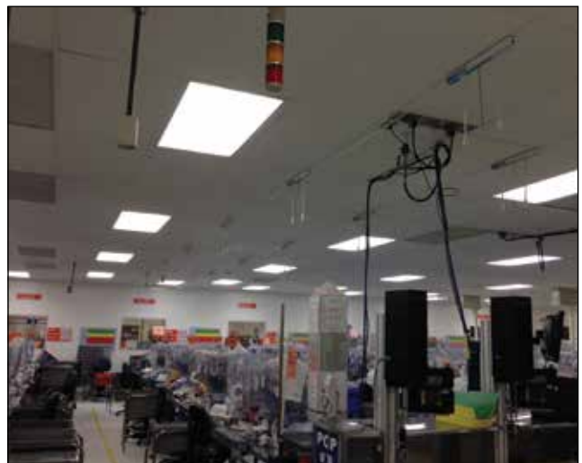
Ceiling Emitters in Production
