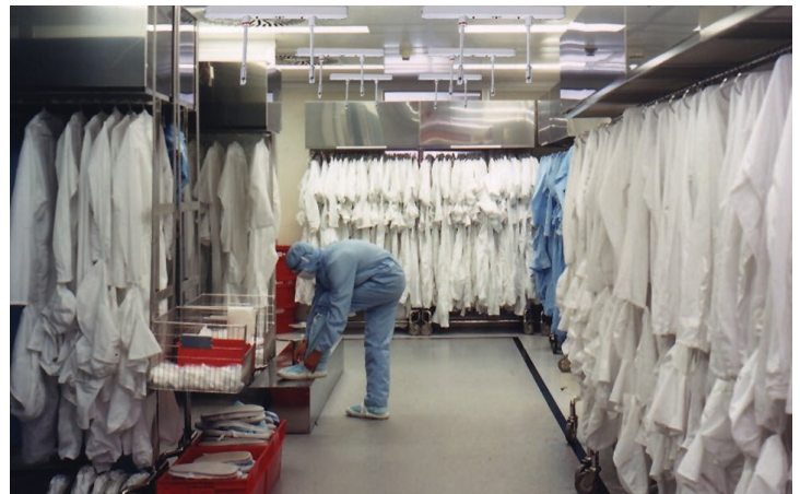
Ceiling Mounted Room Ionization System in Gowning Room
