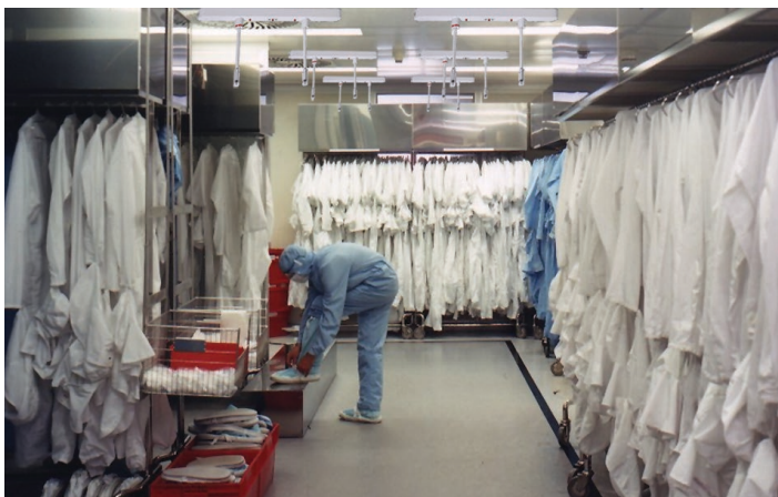
Typical Ceiling-Based Ionization System in Gowning Room
