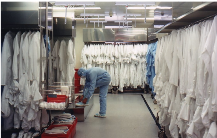
Typical Ceiling-Based Ionization System in Gowning Room
