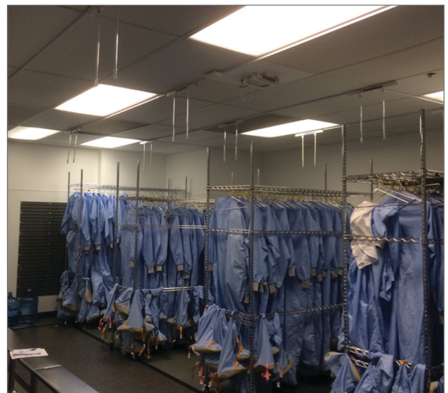
Ceiling Emitters in Gowning Room
