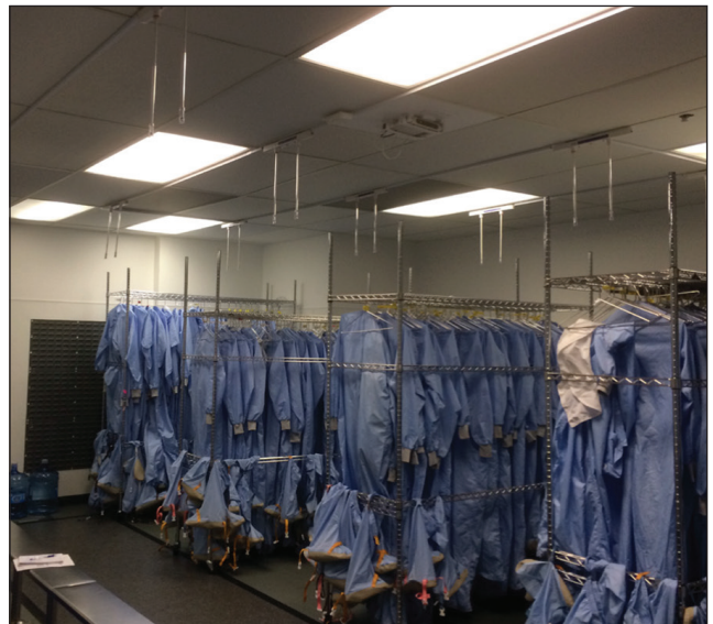
Ceiling Emitters in Gowning Room
